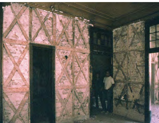
How can another earthquake such as that of Lisbon be withstood? Building in Rua Augusta, 82-84, Lisbon. © Ramon Graus, 1992.
